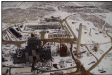
T.S. Power Boulder Valley (Nev.) 200 MW / Jan. 2010
